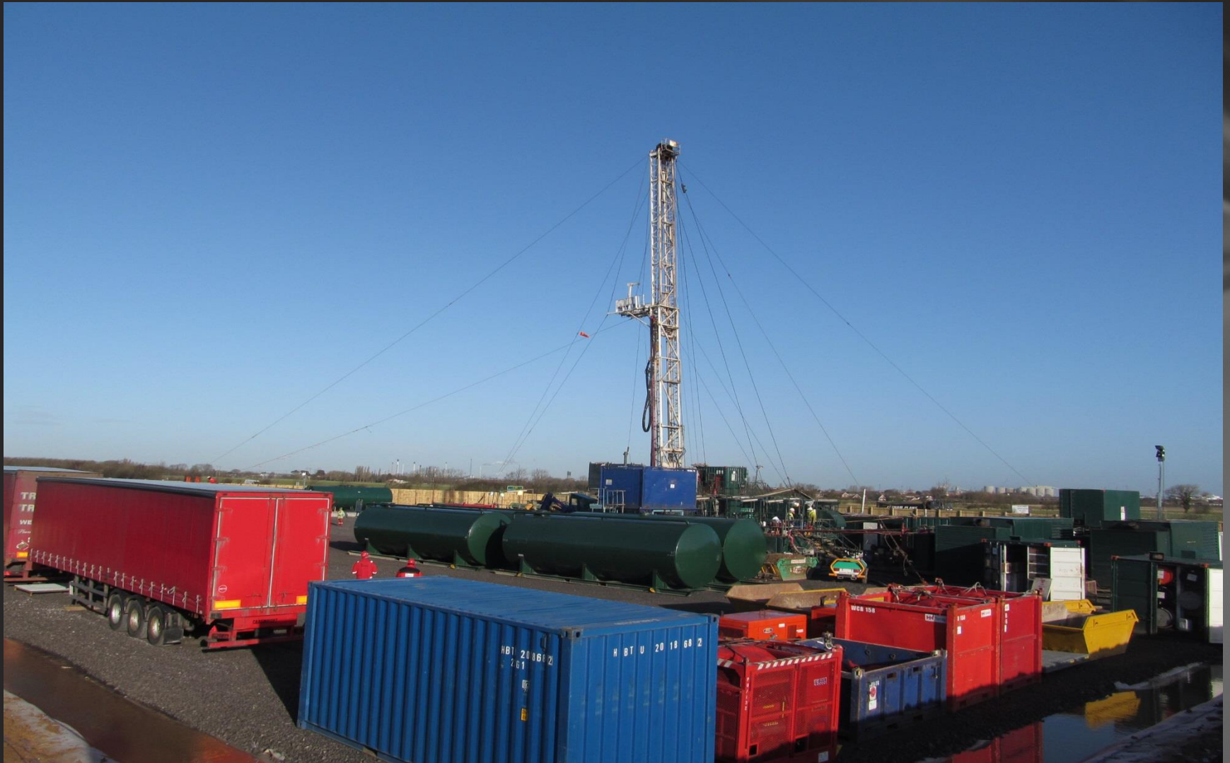
BDF Rig 28 on location and drilling ahead the Kiln Lane exploration well
